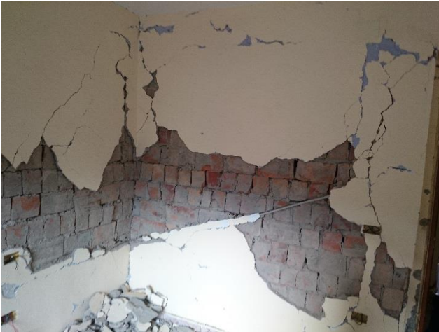
Fig. 5. Poor material quality and workmanship induced failures
