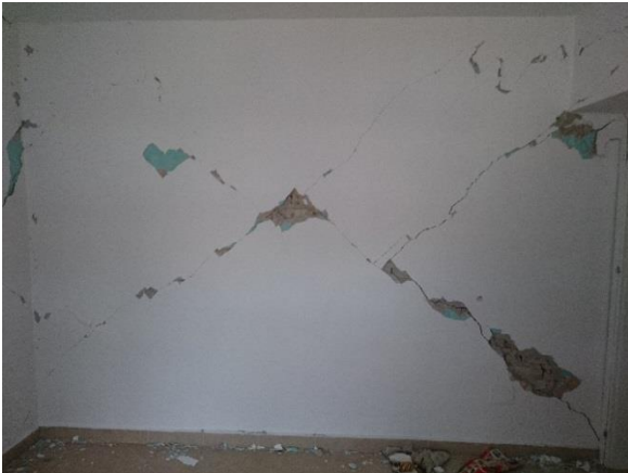
Fig. 1. In-plane shear failure of URM walls
