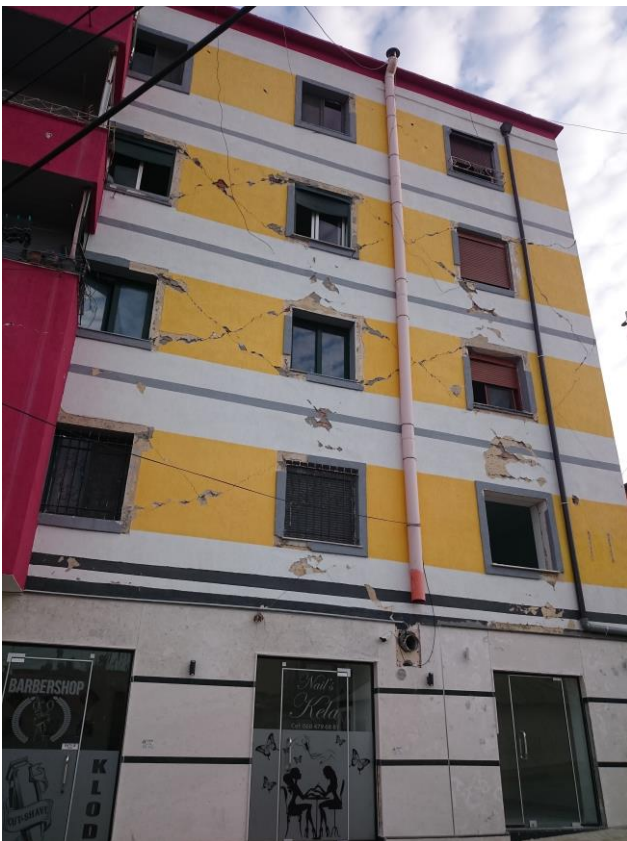
Fig. 2. In-plane shear failure of URM piers
