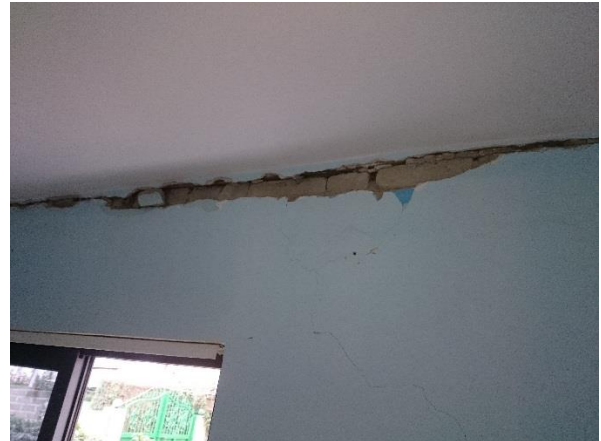
Fig. 3. Failure due to the lack of proper anchorage
